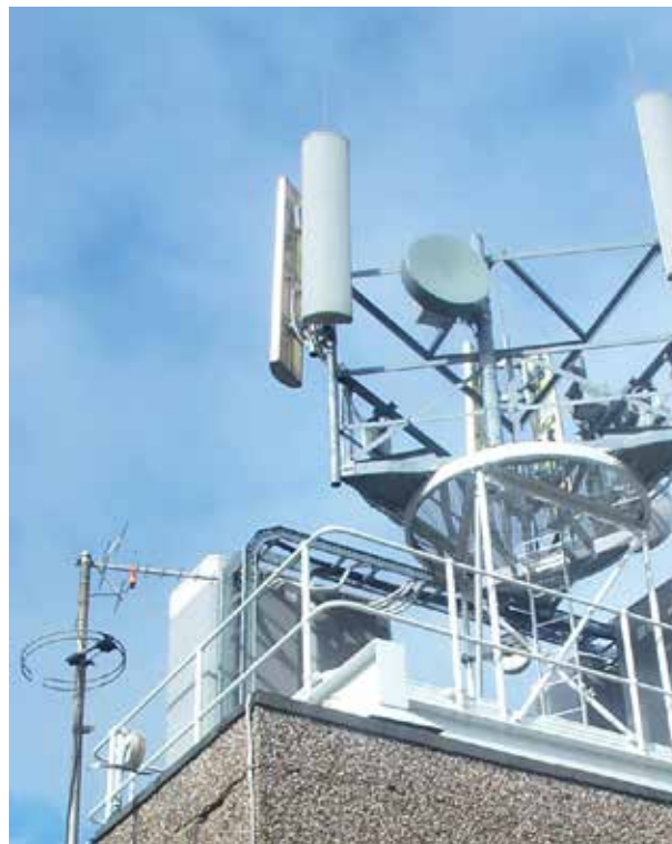
Figure 10.1 — Mobile phone sector antennas and a microwave dish on the roof of the lift house
